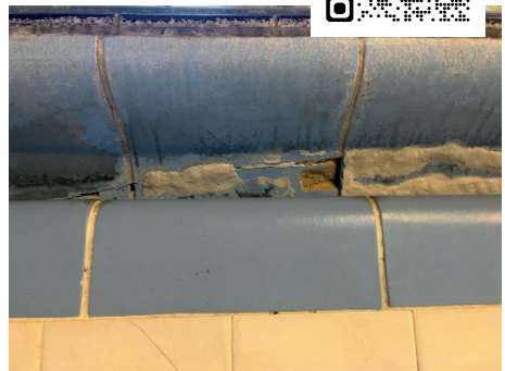
Cracks Observed in the Coping Tiles Near Deep End.
