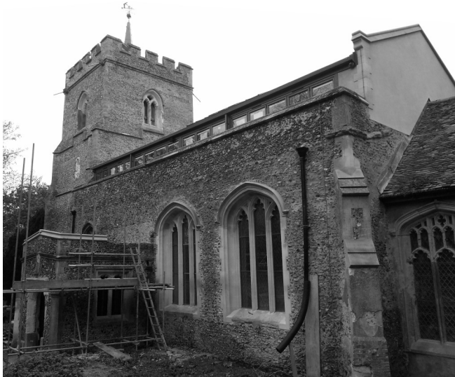
Almost no scaffold here
